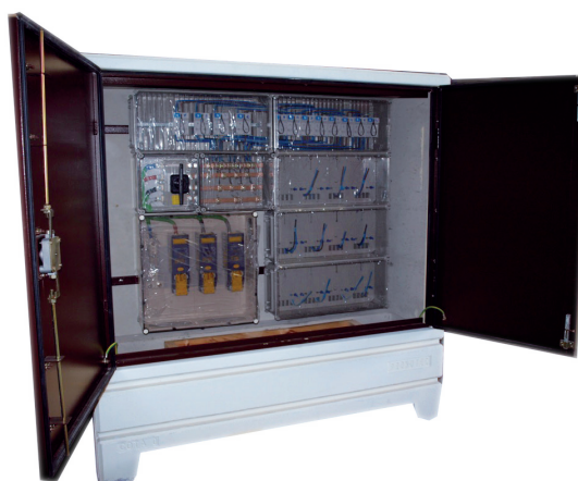
Alumbrado público Street Lighting Cabinets
