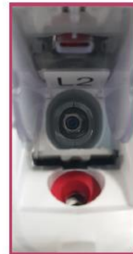
Access to the busbar
